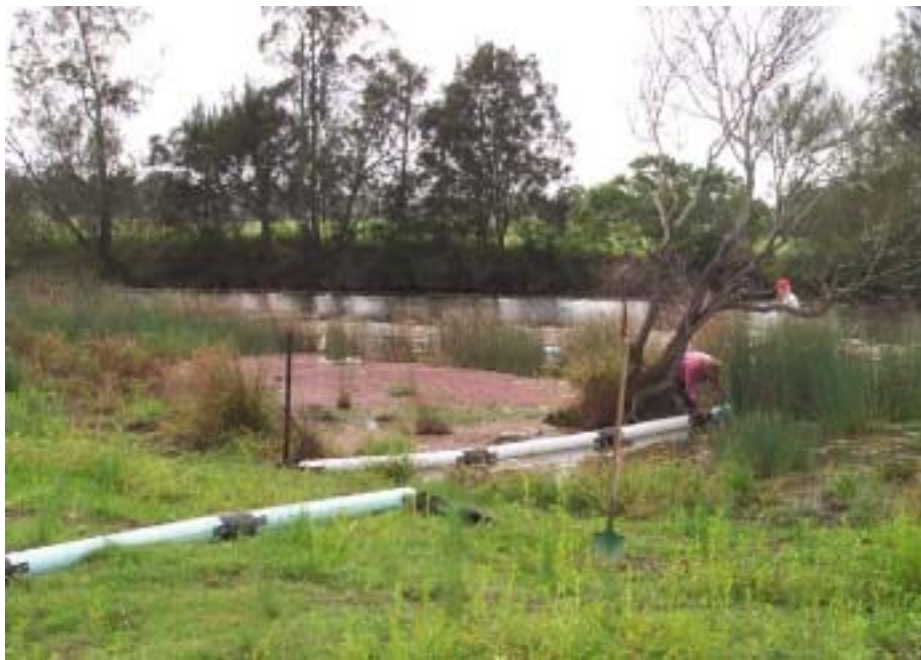
Installing floating Boom at the junction of Williams River and Tumbledown Creek.
